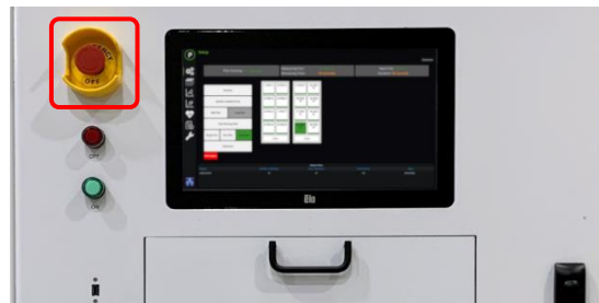
Figure 12: Emergency Stop Switch Location
